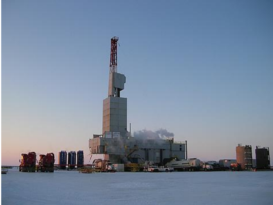
Nordic-Calista Drilling Rig #3 on site at the Ignik Sikumi #1 well, Prudhoe Bay Unit, Alaska North Slope - photo courtesy ConocoPhillips
