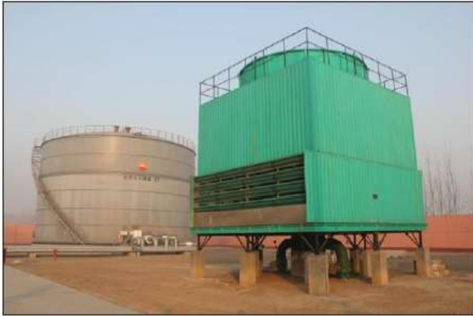
Figure 3. Oil-water tank and cooling tower.
