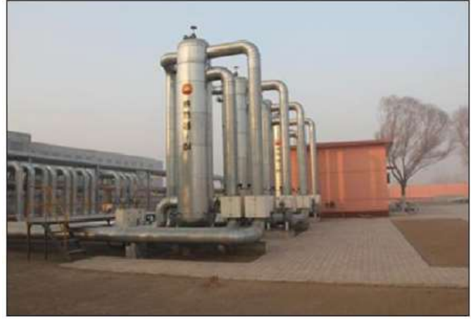
Figure 4. Heat exchanger and geothermal power generation plant.
