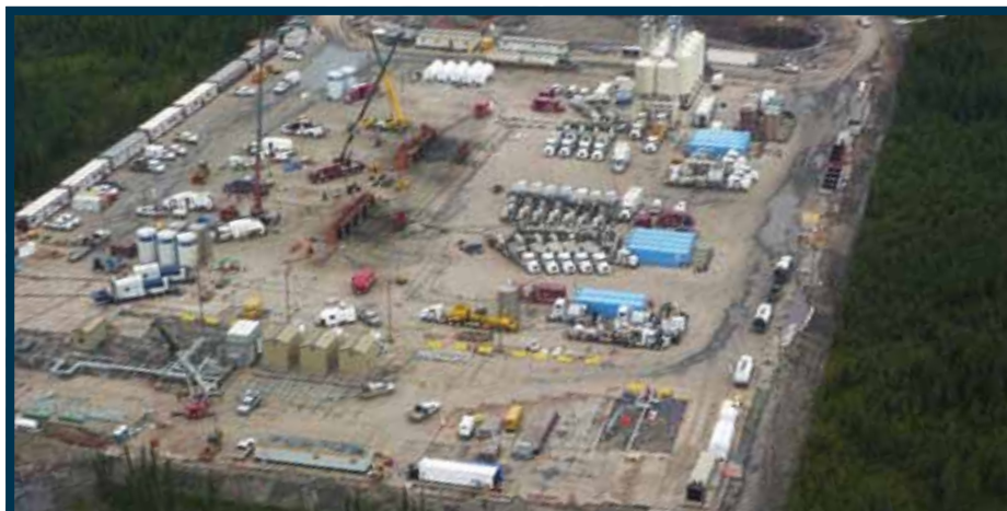
Nexen's summer frac operation in the Horn River Basin; new pipeline construction projects and export facilities in the region could guarantee improved transport of gas to global markets.
